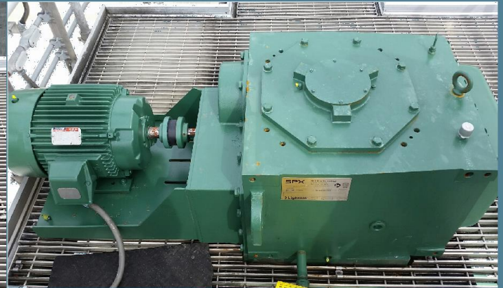
LIGHTNIN GEARDRIVE PRIOR TO COMMISSIONING
